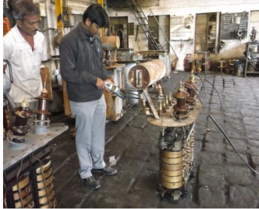
Fig.3. R,Y,B phase test of 63 KVA Transformer
